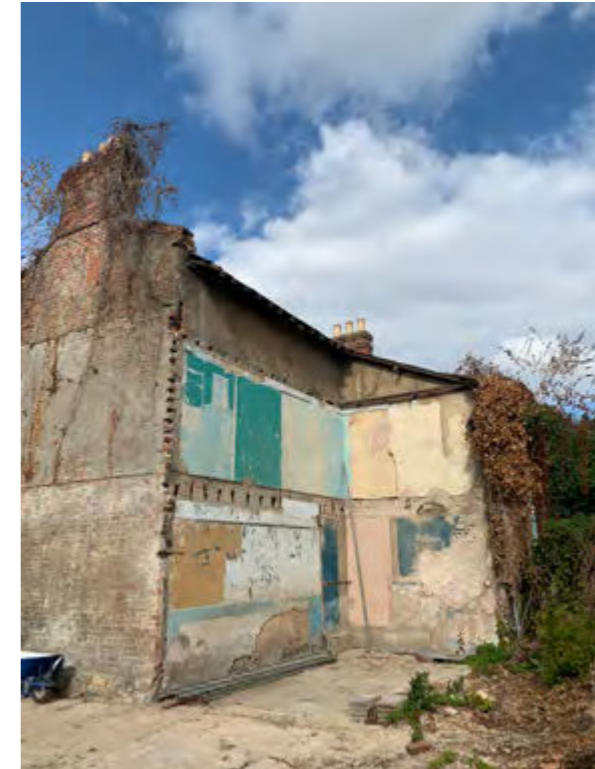
[4] East facing rear facade - This is the section of the building that was altered to give access to the extensions / second dwelling on the site (refer to section 4.0). Situated in this area was a spiral staircase. This section of the building was unsafe / derelict and had fallen into disrepair that required its removal.
