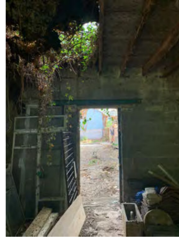
[3] Roof collapse within the outbuilding
