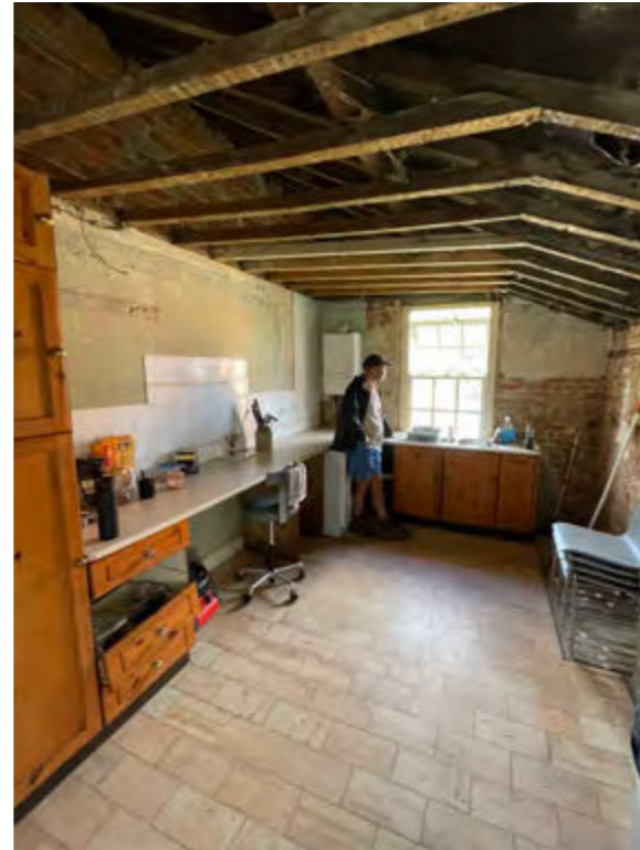
[2] Rear bedroom historically converted into kitchen. Roof structure is compromised by damp and rotting timbers
