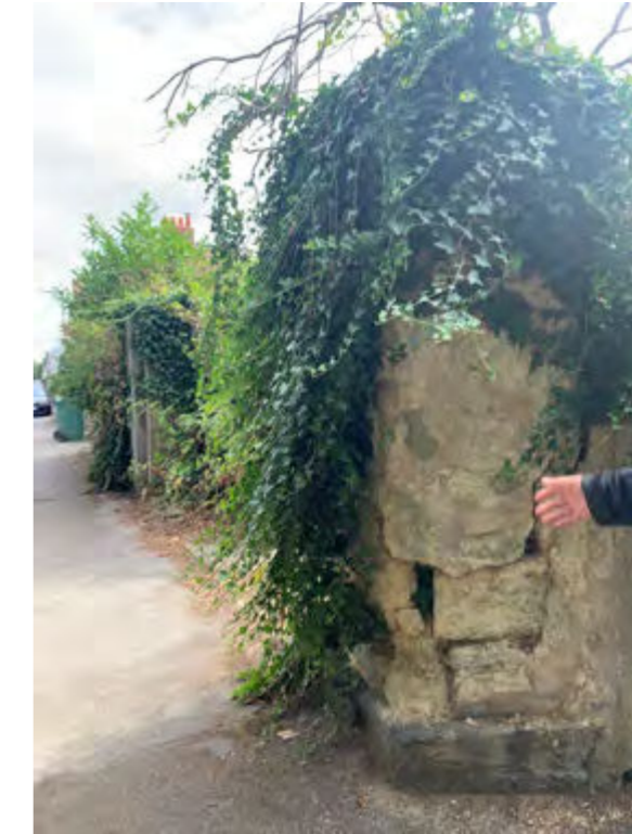
[4] Existing Stone column at the end of Lake street - In need of repair
